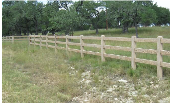
Concrete Rail Fencing
